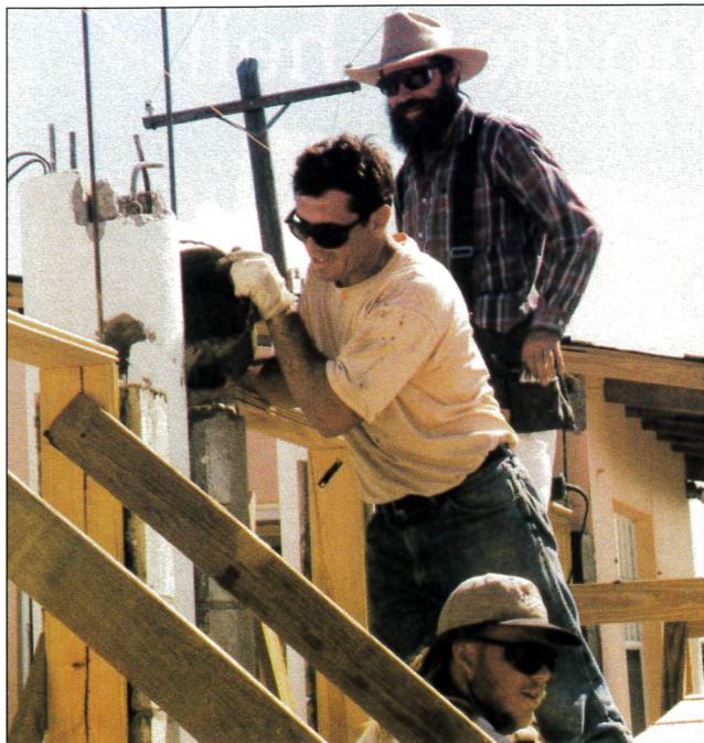
(From top) Randy Baker, Dennis MacDonald, and Jon Sonntag, all from southern California, pour cement to rebuild a wall at Kehl's. "Helping rebuild was nothing compared to the work the mission staff is doing. Those who live and work down here, they're the real story," says MacDonald.
