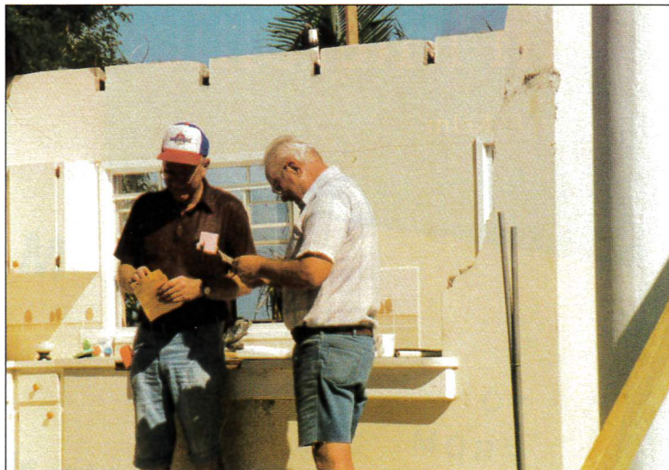
Project manager, Ray Zastrow, and Don Laitinen, a member of Christ the Redeemer, Vt., in Kehl's damaged kitchen. Over 70 people expressed interest in helping with the project, but only 42 were able to help. The type of work and limited housing restricted the number of people who were able to serve.
