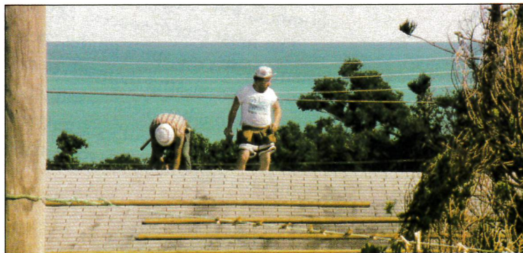
Ralph Pleuss, Manitowoc, Wis., and Kenn Kurtz, Fredonia, Wis., put framing on the roof at the Schneck house. Members of the mission staff went 75 days without electricity and 94 days without phones at their homes. The only working phone was at church. "When you see what these people went through, you know why we're here," says Kurtz.
