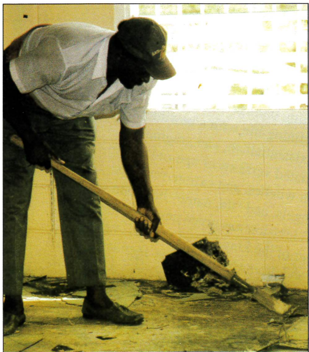
St. John member, Wilbert Richards, rips up floor tiles in one of the preschool classrooms. The classroom is now tiled and painted, but not yet reoccupied. By using volunteers from the church and from around WELS, Builders for Christ saved over $100,000 on repairs.
