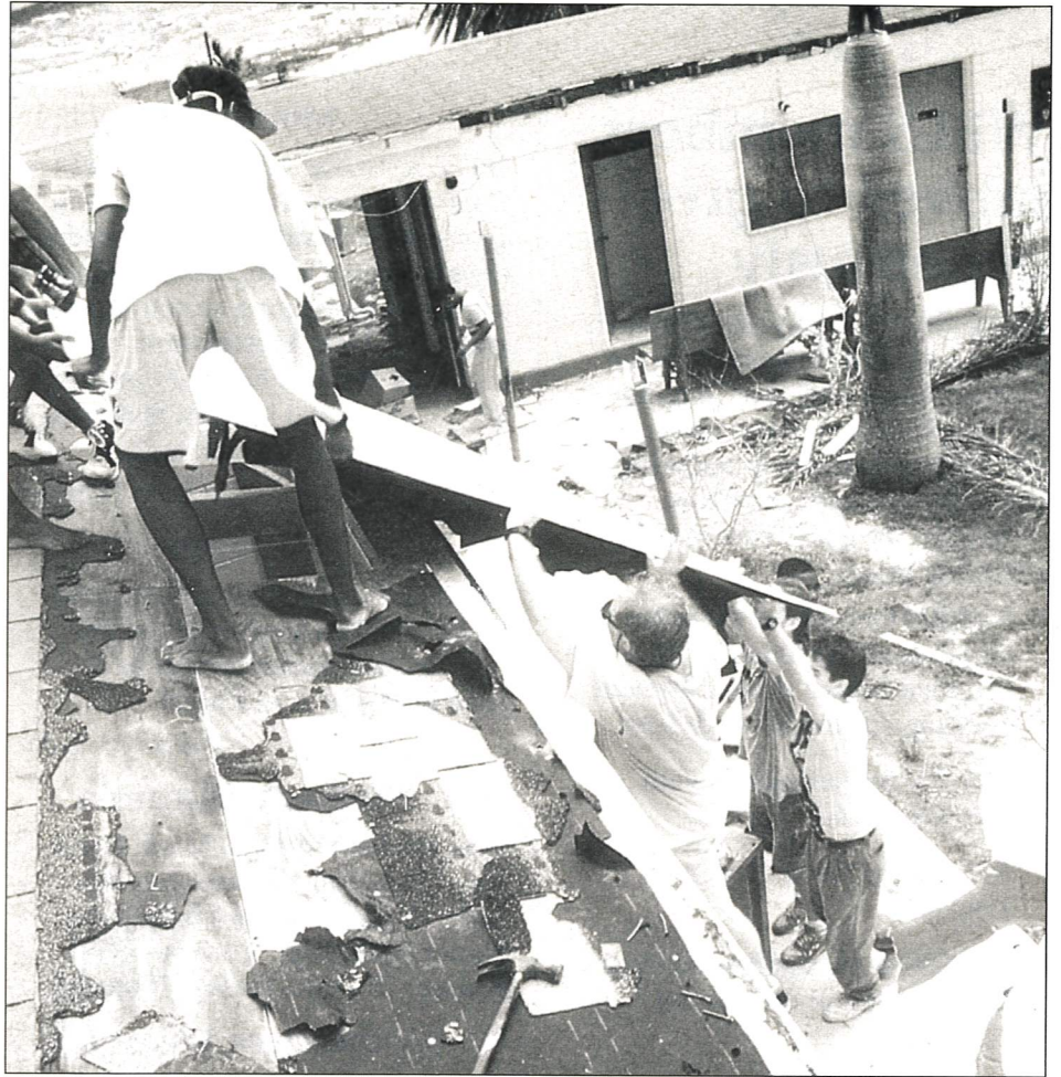
Members and mission staff of St. John's work to repair holes in the school's roof. Over 24 people showed up to help restore the school, even before repairing their own homes.
