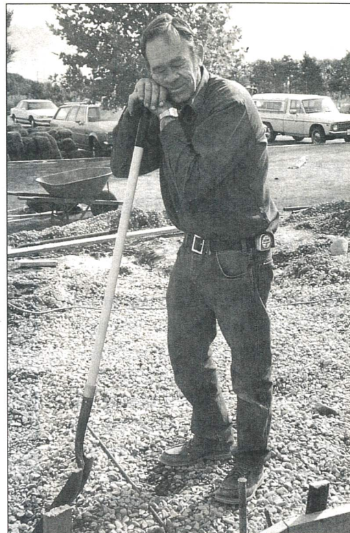
Don Homann takes a break while working on Prince of Peace’s new education and fellowship wing.
