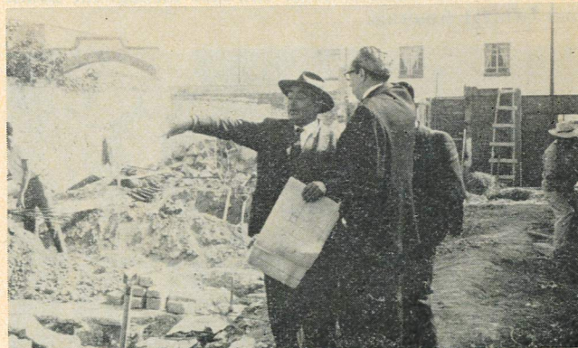
The contractor points out progress in the construction of our chapel in Mexico City to Pastor David Orea Luna. Groundbreaking services for the beginning of construction were held on December 14, 1969. The chapel should be completed by June.
